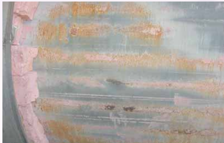
Insulation removed from a pipe originally coated with a zinc containing coating. Zinc has worked but by sacrificing, thus limiting the lifetime of the protection.
